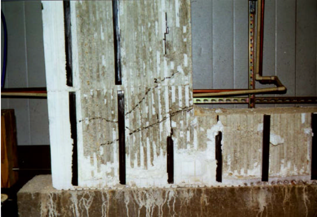
Figure 3 Typical Hairline Cracking at the Corners of the Window Opening
