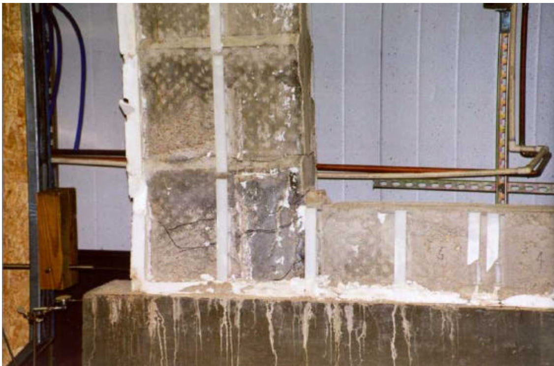
Figure 8 Typical Hairline Cracking at the Corner of the Window Opening (Waffle No. 2)
